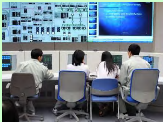
Nuclear Power Training Center Ltd.
