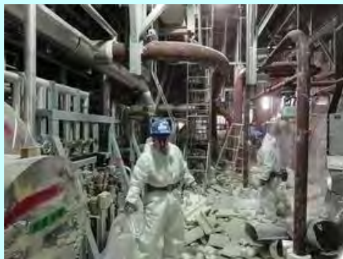
Demolition work site of a nuclear power plant decommissioning (Fugen Power Station)
