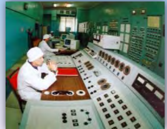
IGR- Research Reactor console
